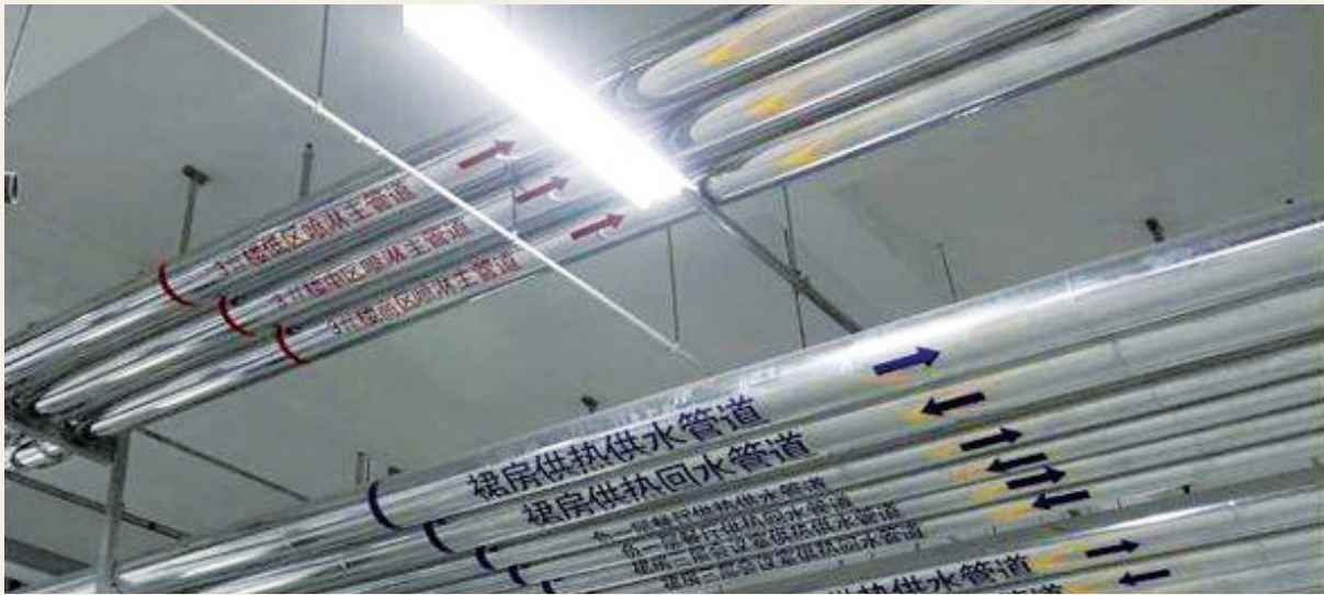
Illustration of the pipeline marking
