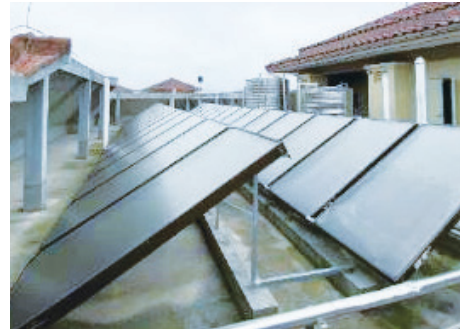
Solar water heating system
