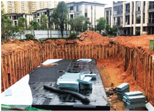
Rainwater recovery system
