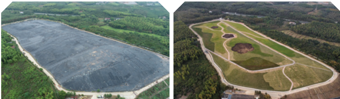
Guangde Household Waste Landfill Restoration and Closure Project — before and after restoration
